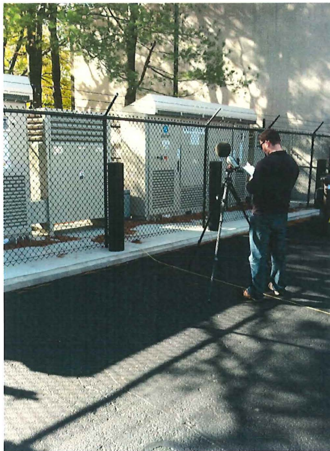
Figure 2. Sound Level Meter on the Axis Perpendicular to the Face of an Inverter at a Solar Photovoltaic (PV) Array
